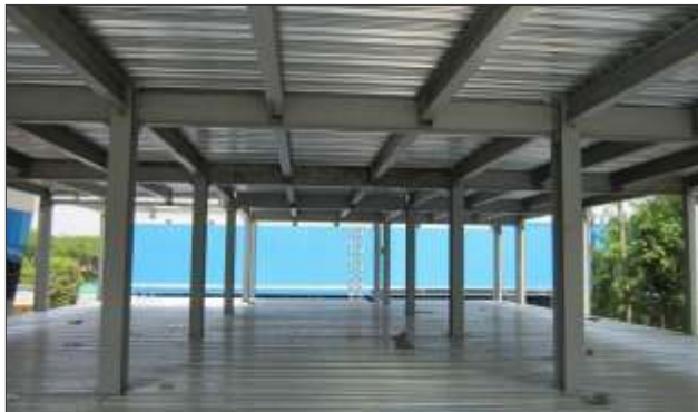
VOLVO EICHER MEZZANINE FLOOR
