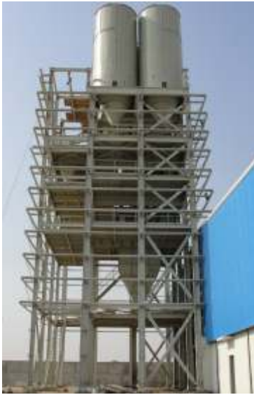
MULTI STOREY STEEL STRUCTURE FOR HEAVY DUTY SILOS
